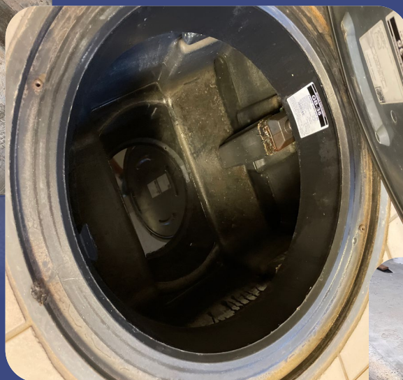
Empty Grease Trap
