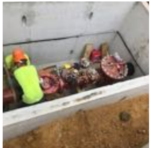
Image from one of our Large Meter and Large Meter Vault Replacement project sites in Prince George’s County.
