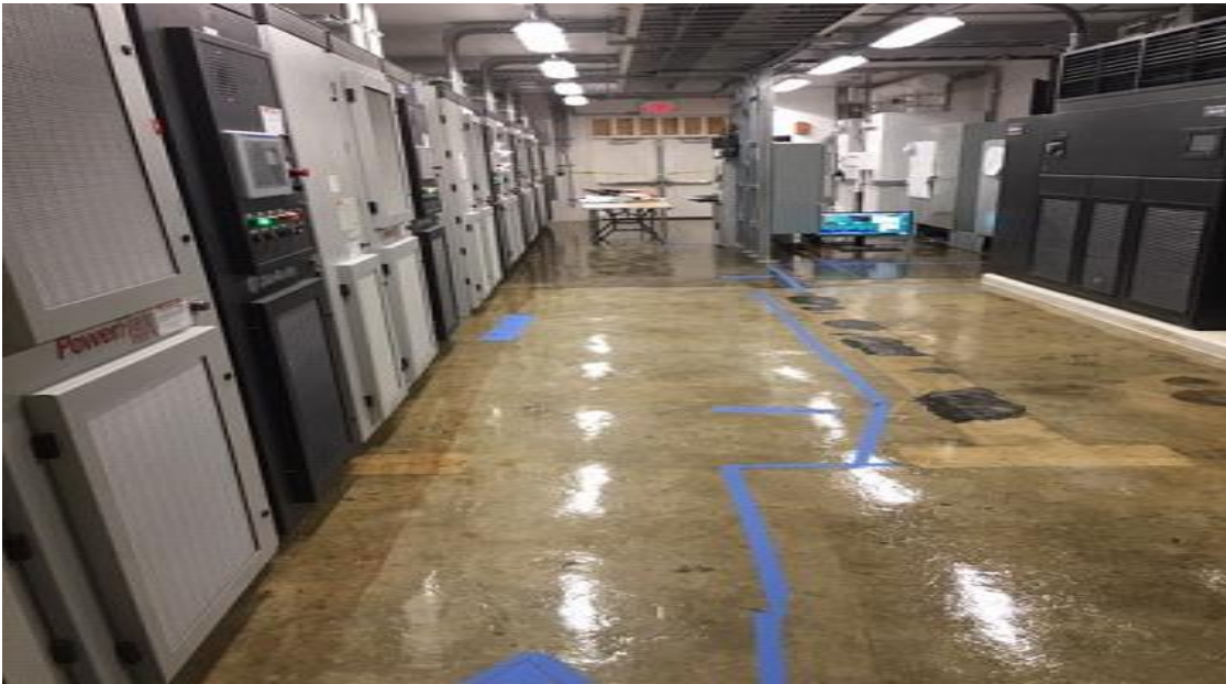
Interior of New Electric Room
